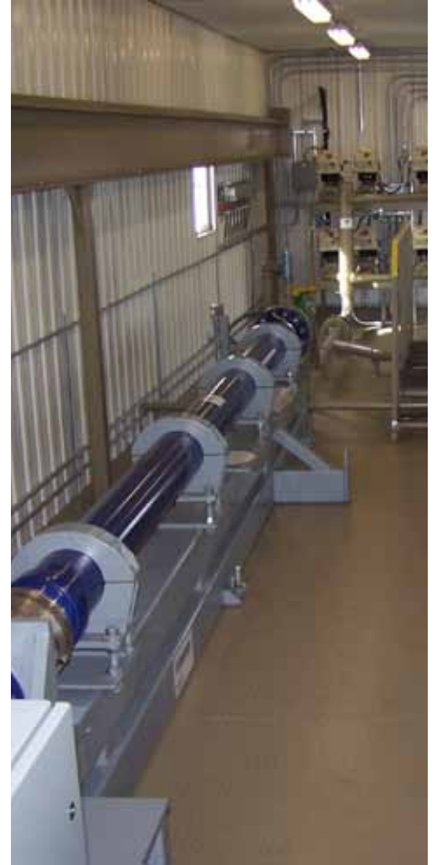
RedaHPS system installed at Double Eagle Petroleum's Catalina Unit.
